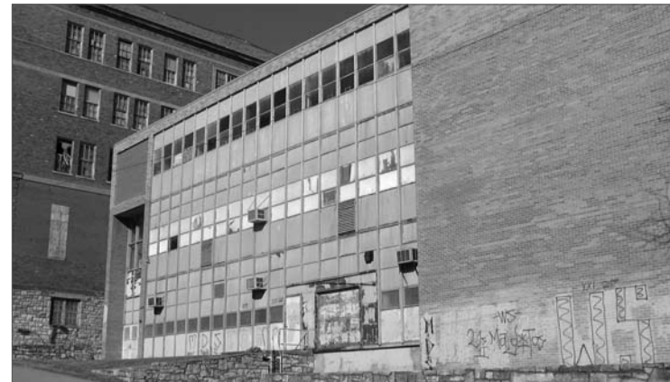
The West Junior High complex has been a cause of disagreement for years between Westside residents and the KCMO School District. The Board has decided to rid itself of the problem by auctioning the property.
